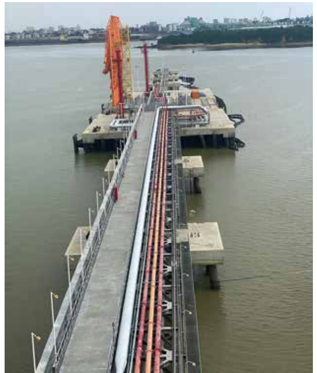
Kipevu Oil Terminal 2, Mombasa Kenya
