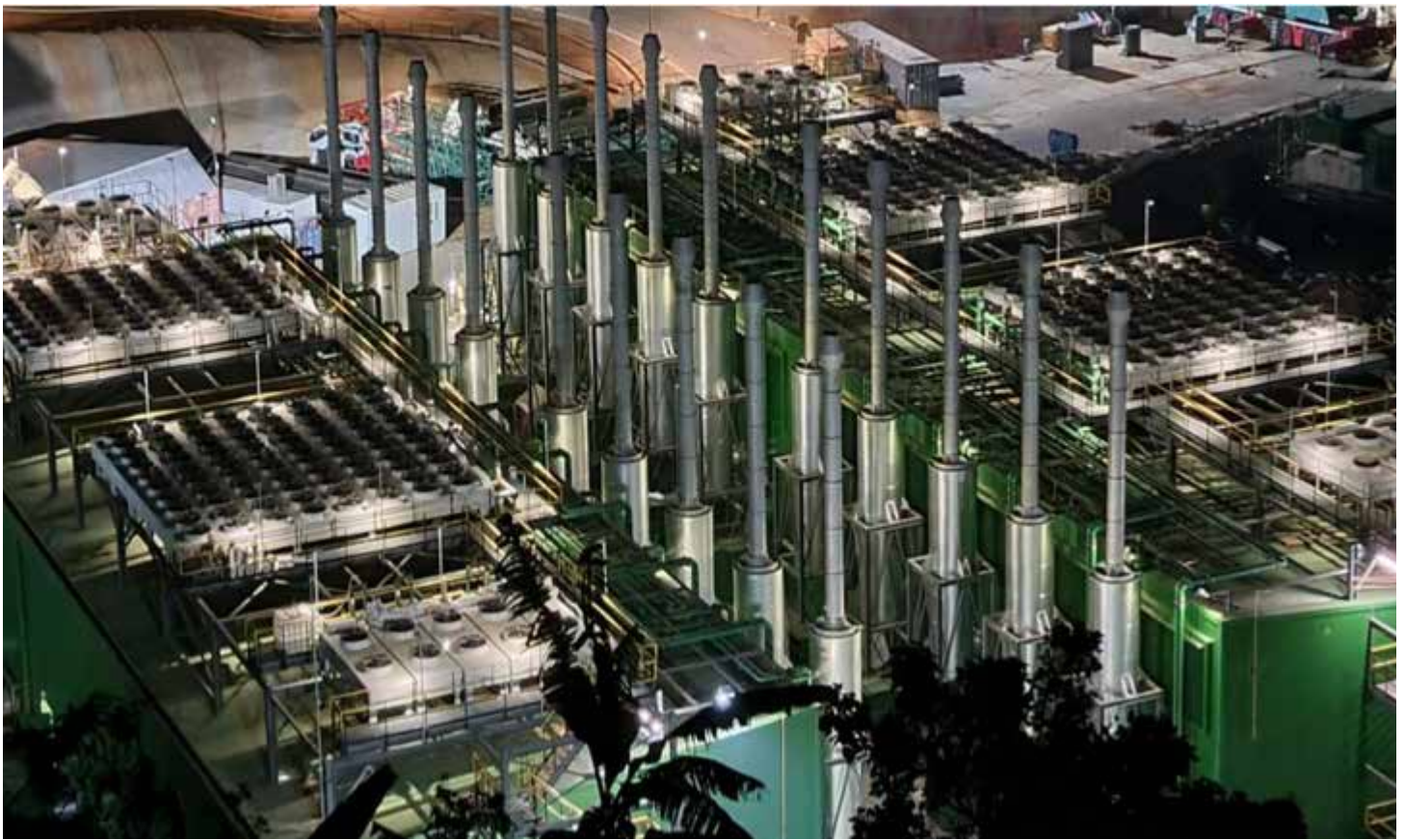
Shema Power Plant on Lake Kivu
